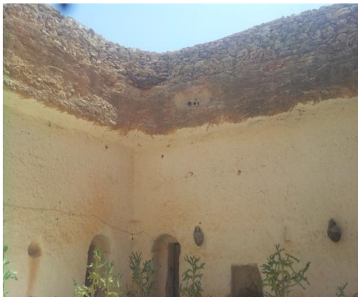
Figure 8.32: The lack of a roof over the courtyard.
