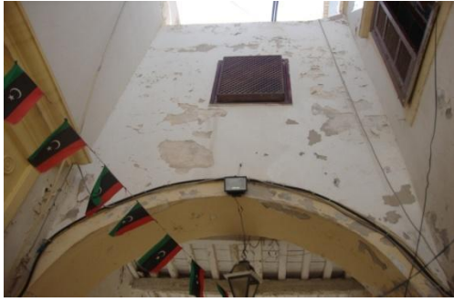
Figure 6.1: Sabat is built between one house and another in the old city of Tripoli.
