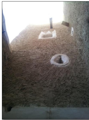
Figure 8.53: Openings in the ceiling alleys for air circulation.
