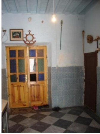
Figure 8.8: The Sakifa or the corridor with ceramics for adornment in Mahmoud Sola house in Tripoli.
