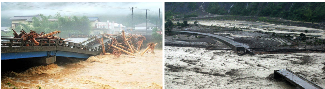
Fig. 1.3 Bridge failures during the typhoon Morakot, Taiwan, 2009
