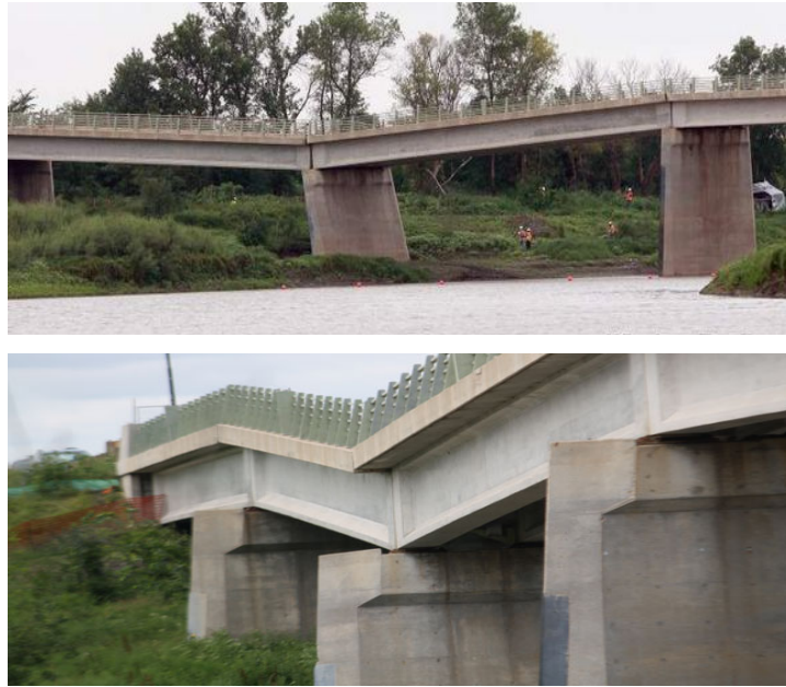
Fig. 1.10 Failure of the St. Adolph Bridge, Winnipeg, Canada, 2009
