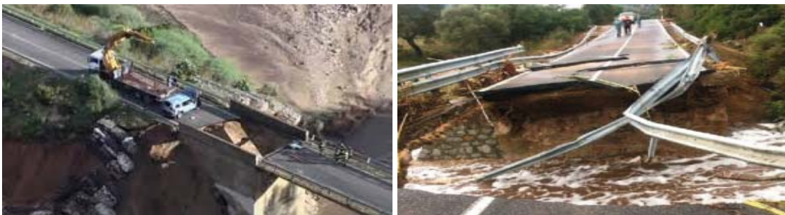
Fig. 1.14 Bridge failures near Dorgali (left) and Olbia (right), Sardinia, 2013
