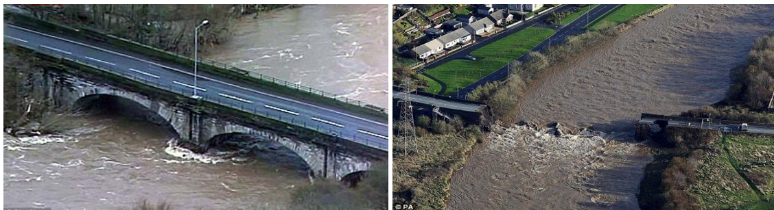
Fig. 1.7 Northside Bridge prior and after the failure, Workington, UK, 2009
