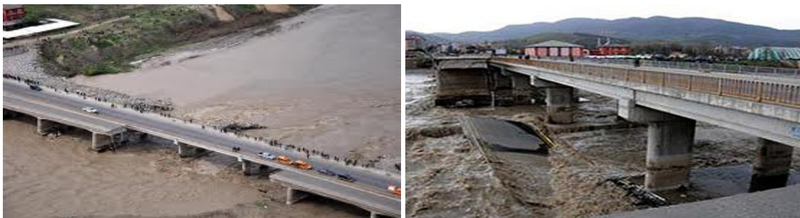
Fig. 1.11 Failure of the bridge on the river Filyos, northern Turkey, 2012
