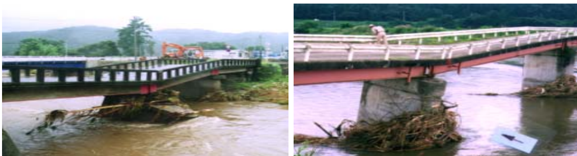
Fig. 1.1 Bridge failures in the Kanto region, Japan, 1998, [Fukui and Nishitani, 2002]
