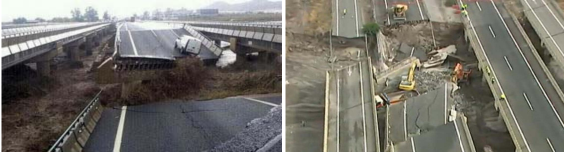
Fig. 1.12 Failure of the bridge across Rambla de Béjar, Spain, 2012
