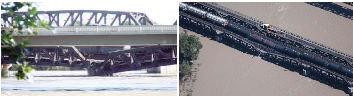
Fig. 1.13 Bonneybrook bridge collapse in Calgary, Canada, 2013
