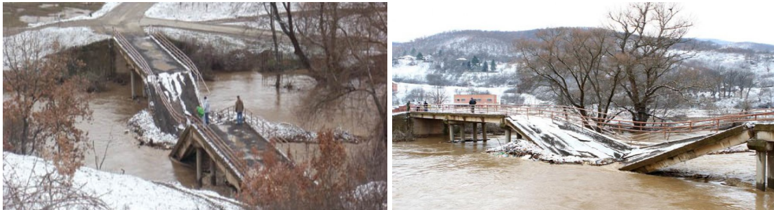
Fig. 1.15 Bridge failure, Lešak, southern Serbia, 2013
