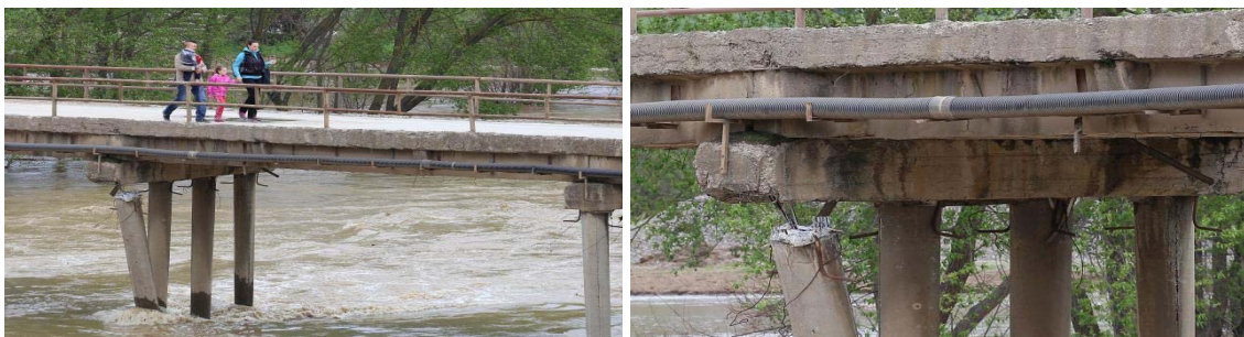
Fig. 1.17 Damaged bridge pier, Lešak, southern Serbia, 2014
