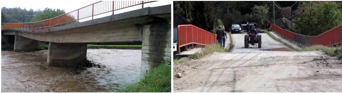
Fig. 1.18 Bridge failure, Topola, central Serbia, 2014.
