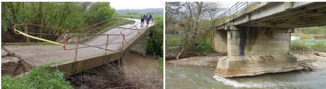
Fig. 1.16 Bridge failure near Kraljevo (left) and scour-critical bridge near Vranje (right), Serbia, 2014
