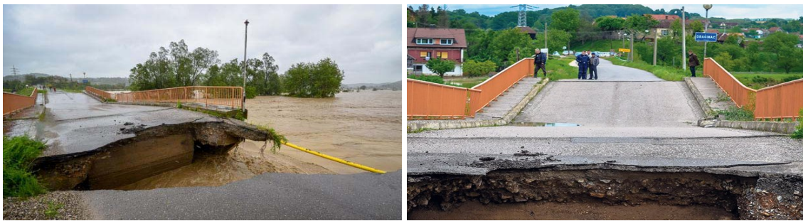
Fig. 1.19 Bridge failure, Draginac, central Serbia, 2014.
