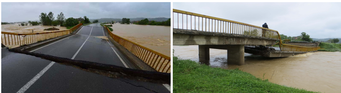
Fig. 1.20 Bridge failure, Koceljeva, western Serbia, 2014.
