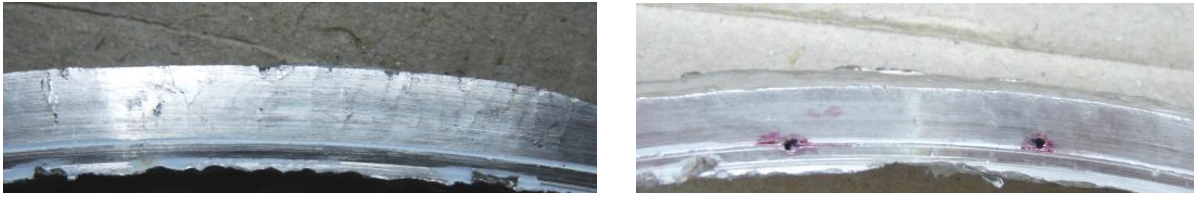
Figure 1-7. Cross section views: a) network of cracks, b) pores on inner side
