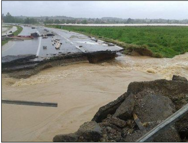
Figure 6. Damaged road near town of Koceljeva in the Tamnava River valley during the May 2014 flood (source: Koceljeva municipality web site 2 )
