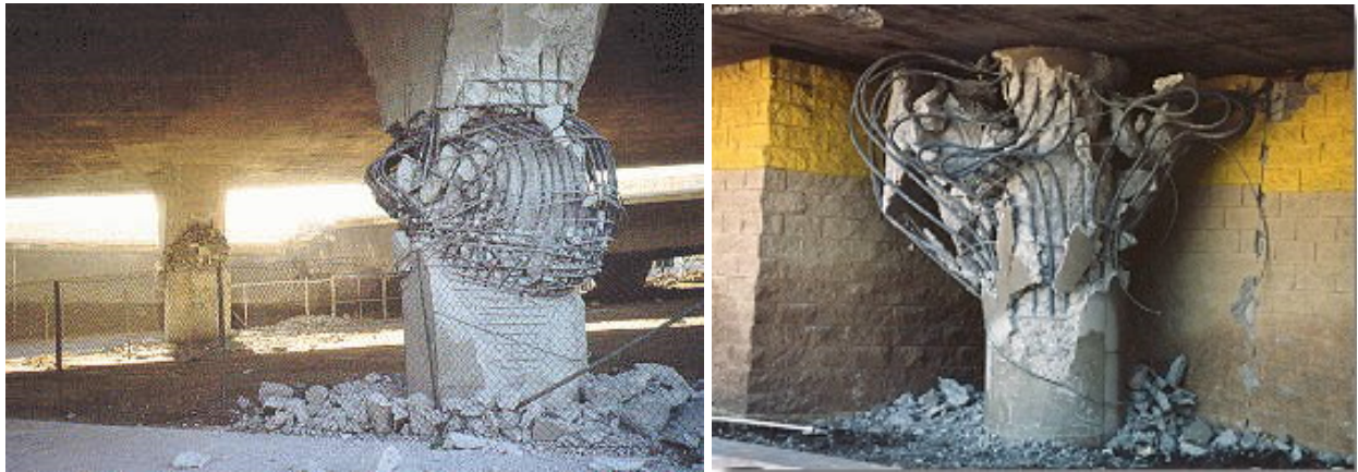
„Northridge Earthquake“, 17. januar 1994., Kalifornija, SAD, Magnituda 6,8 http://www.whatiscivilengineering.csce.ca/structural_earthquakes.htm
