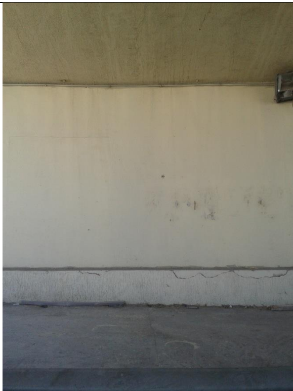
Figure (IX-31): View of supporting wall, damages of plinth
