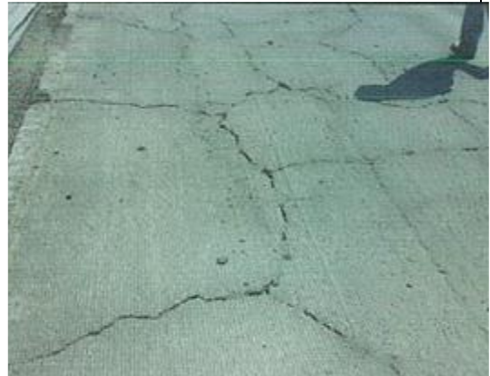
Figure (VIII-38) Cracks in down layer, after cleaning
