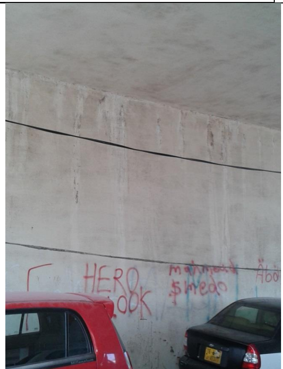
Figure (IX-82) View of abutment, leakage through horizontal crack
