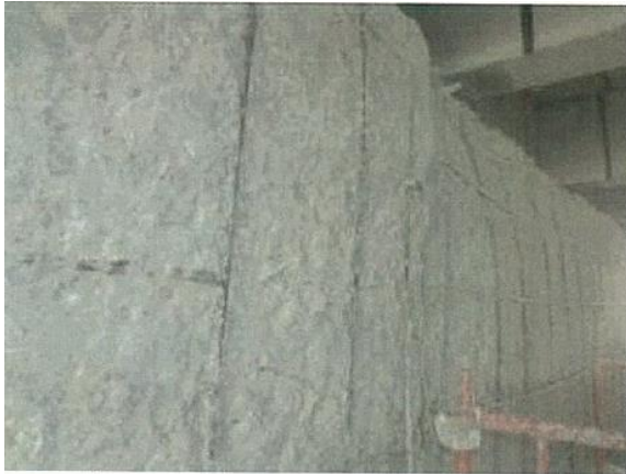
Figure (VIII-186) The view of abutment after removal of all damaged concrete
