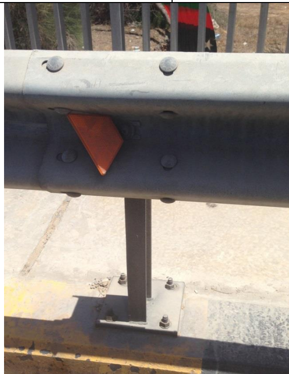
Figure (IX-21) A general view of reflective sign in guardrail
