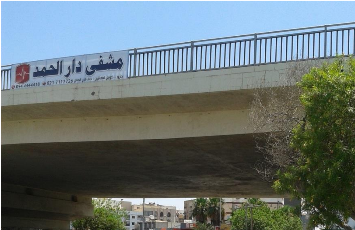
Figure (IX-71) View of cantilever slab, vertical and horizontal cracks
