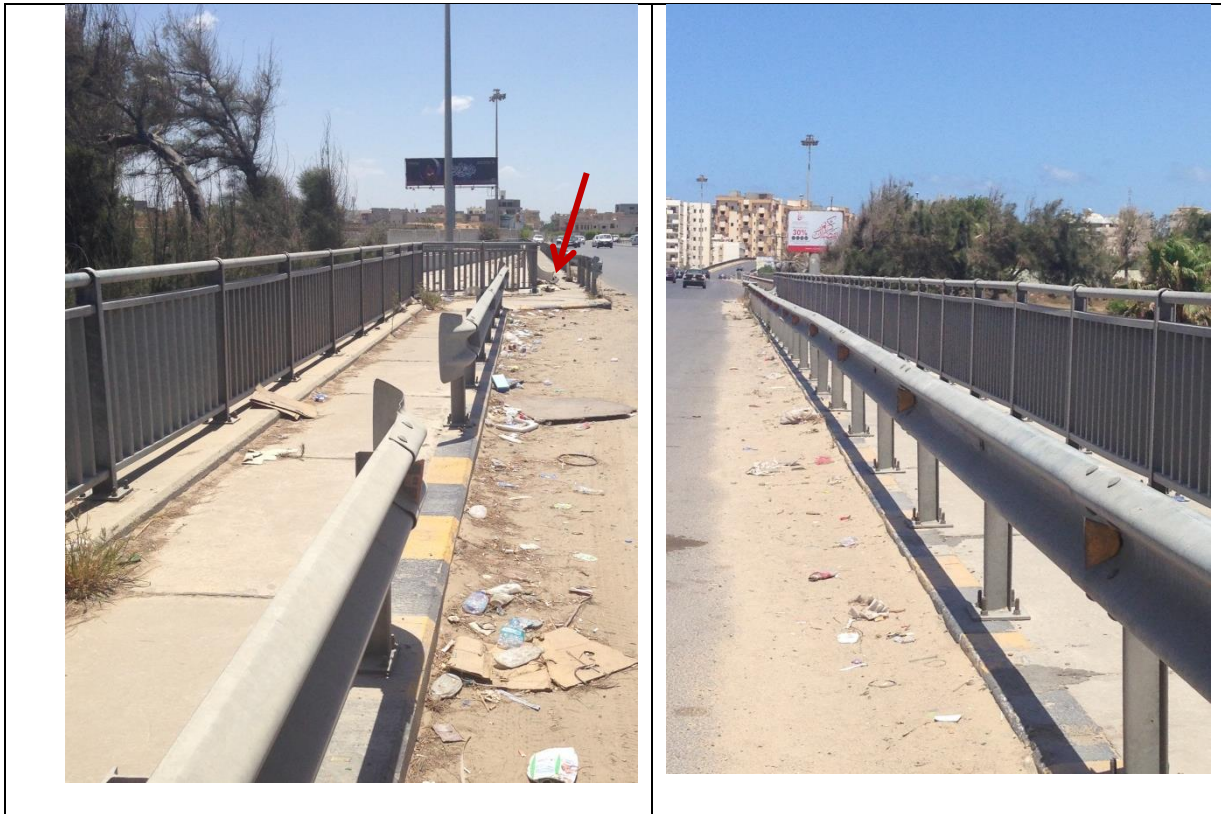
Figure (IX-19) General view of the guardrail on the bridge with the missing of part of it
