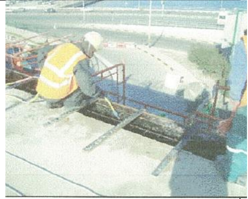
Figure (VIII-171) The new RC beam for fence: casting of concrete in framework
