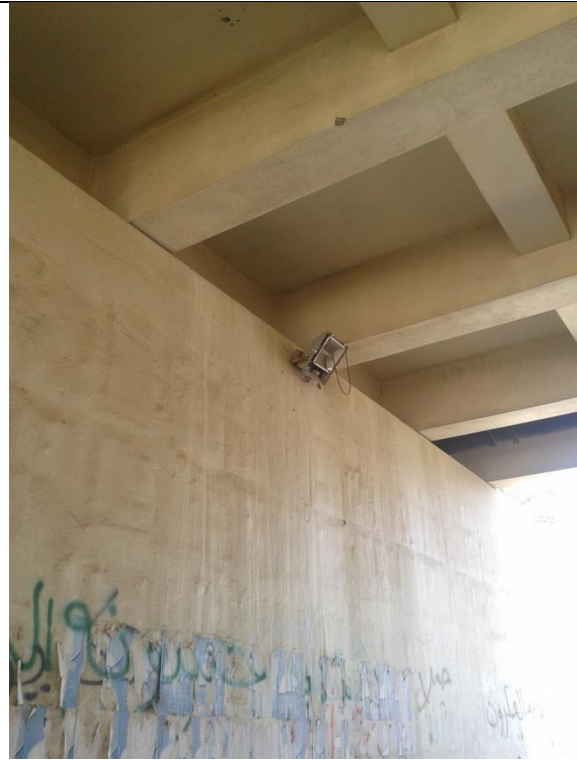
Figure (IX-139) Uneven concrete surface of an abutment, in detail
