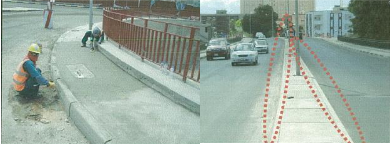
Figure (VIII-88) New side walk with new curbstone and casting of new catch pit
