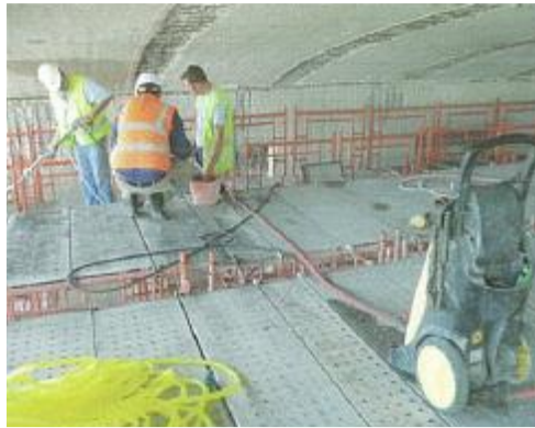
Figure (VIII-5): Cleaning the surface of concrete after removing concrete cover by water jet machine
