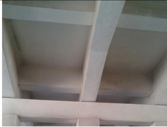
Figure (IX-144) A general view of down part of deck slab in superstructure of bridge
