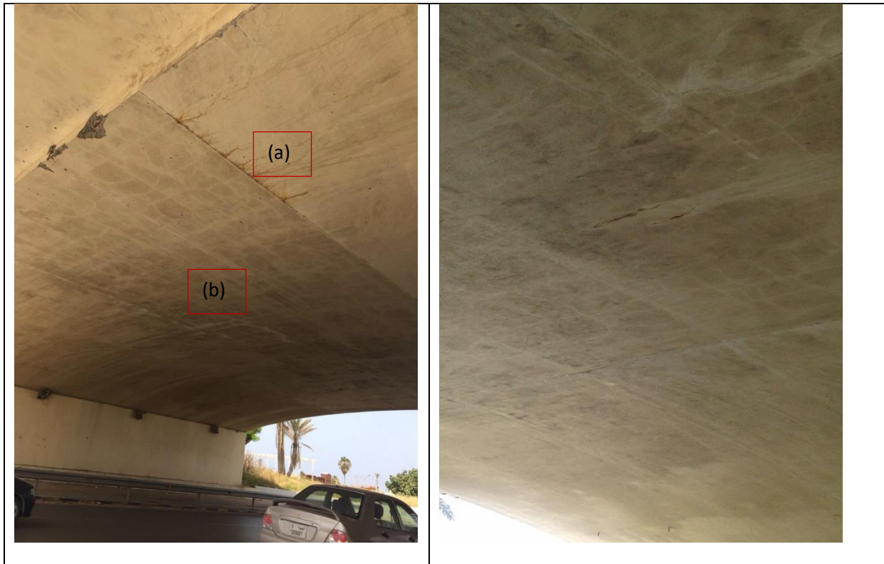
Figure (IX-27): View of deck slab with abutment, (a) rust stains, (b) white stains
