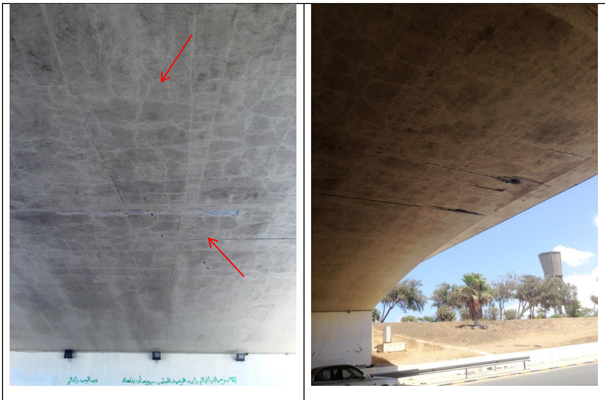
Figure (IX-9) Net like cracks, local spalling off of repair mortar (cover) and shallow cut “channels” on down side of bridge deck slab.
