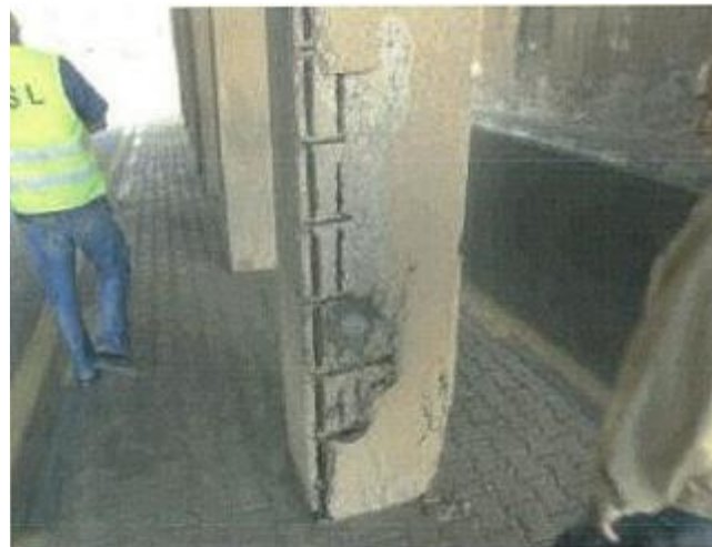
Figure VI-162. Damaged column: A large delamination and spalling off of cover, Exposed corroded reinforcing bars
