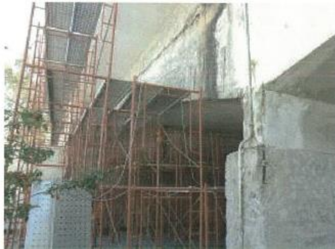
Figure VI-107. Dark traces of leakage water on lateral beam
