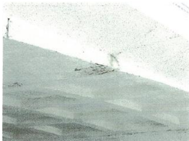
Figure VI-83 Ceiling, Local honeycomb, visible corroded bars
