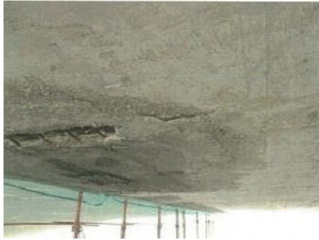
Figure VI-27. Deck ceiling slab: corrosion of rebars, delamination and falling down of deck ceiling cover, wet stains
