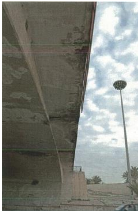
Figure VI-52. Cantilever slab and part of the ceiling deck; falling off painting and plaster layer, white and dark stains along the edge of slab, damage of concrete due to corrosion of reinforced bars
