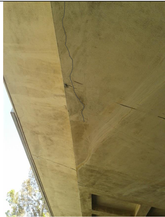
Figure (IX-47) Crack along the edge of lateral beam, water traces
