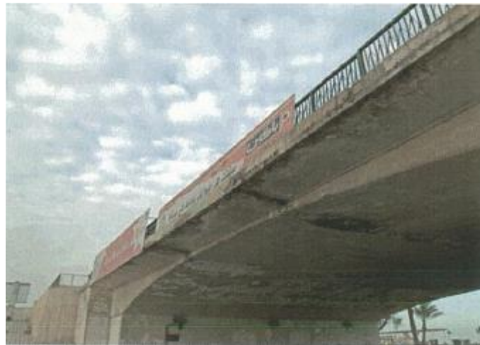
Figure VI-54. Cantilever slab and deck ceiling slab; the largest damage in the centre of these elements
