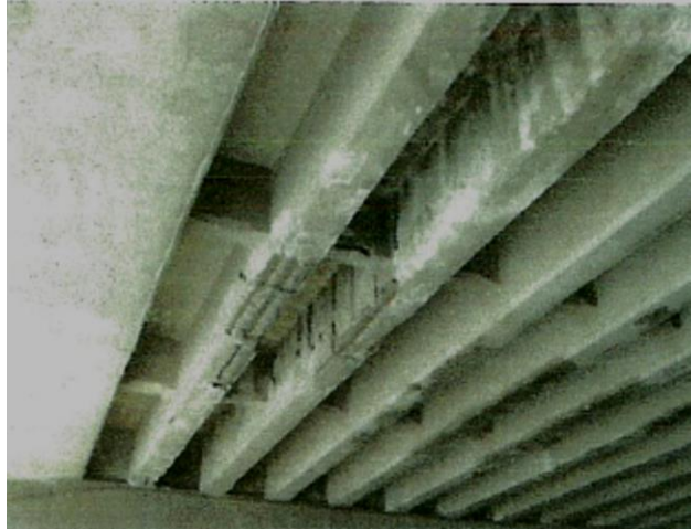
FigureVI-148. Exposed reinforced bars in slabs beams
