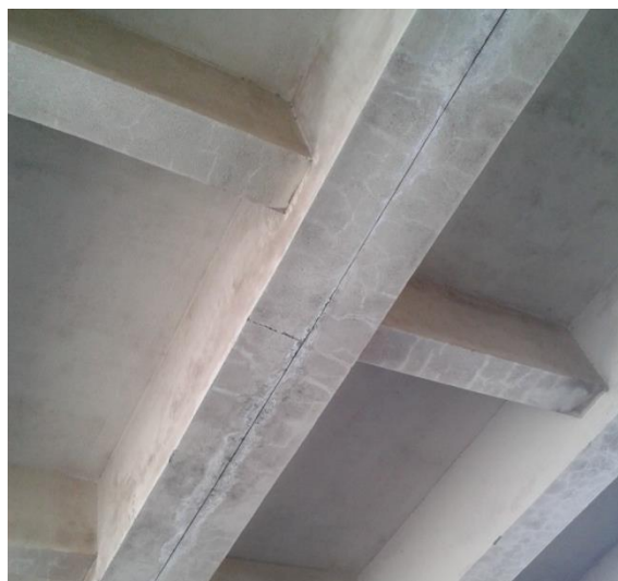
Figure (IX-96) Expansion joint in superstructure of the bridge: water leakage, white stains
