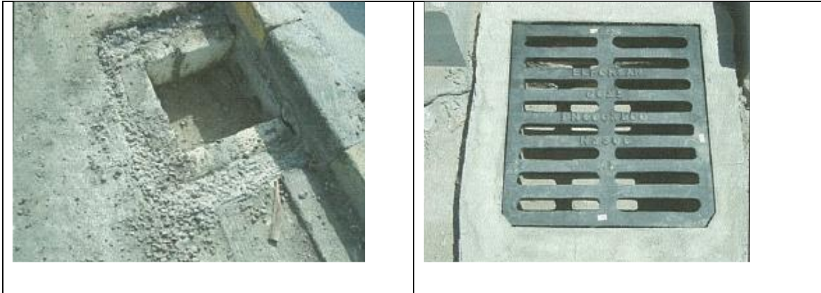
Figure (VIII-34). Detail of cover for box of valve and catch pit after finish
