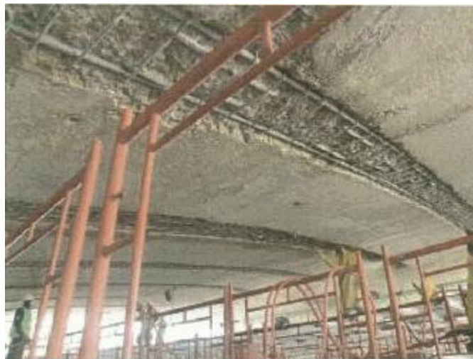
Figure (VIII-13) Covering the rebars on ceiling beams with cementitious base protection
