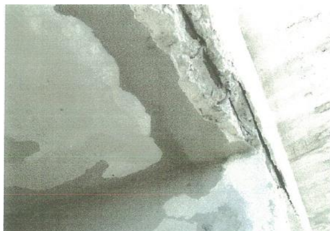
Figure VI-55. Detail of ceiling slab: falling off painting and plaster layer due to bad adhesion and concrete cover caused by corrosion of bars
