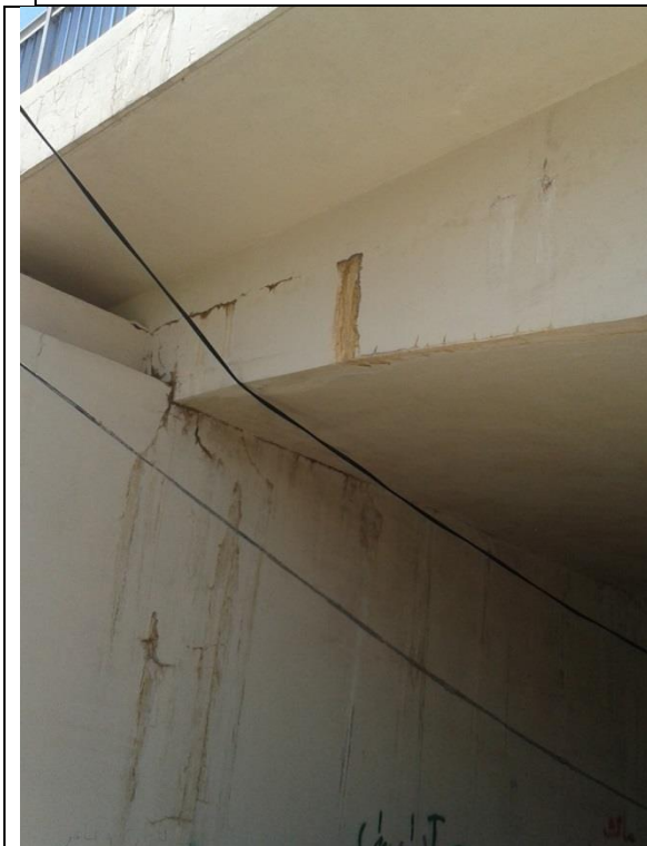
Figure (IX-81) View of external part of abutment, cracking of wall
