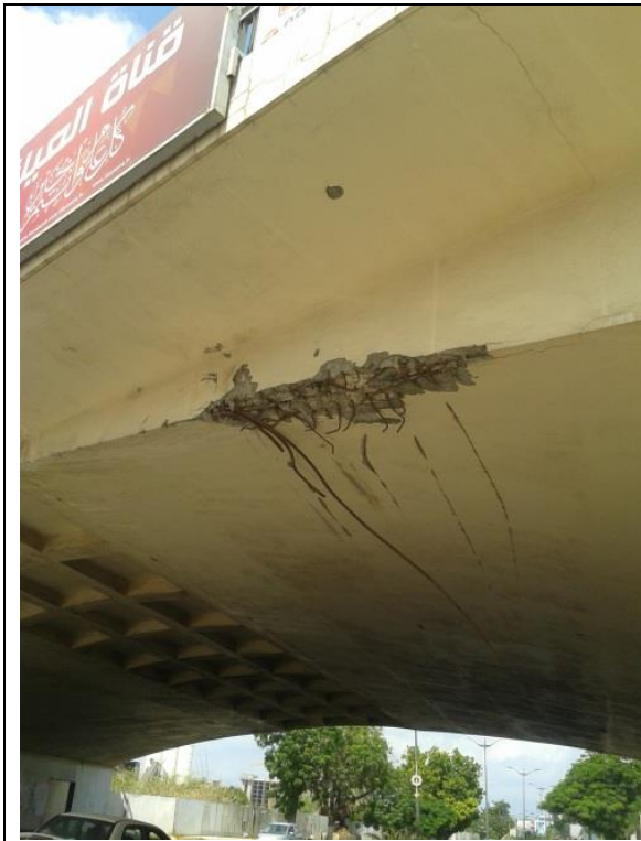
Figure (IX-46) Mechanical damage of lateral beam
