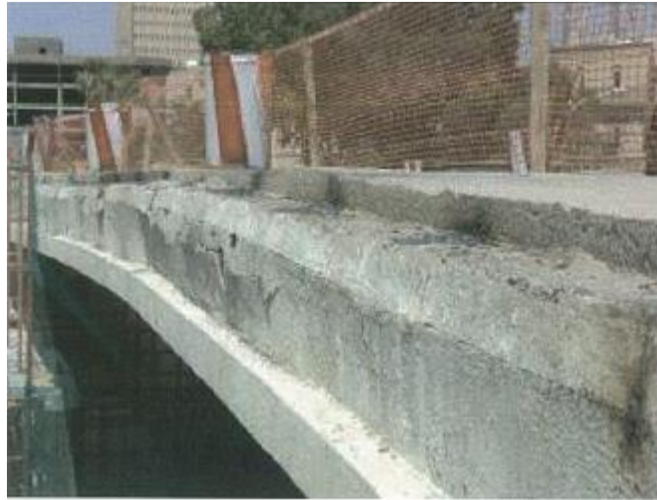
Figure VI-106. View of damaged cantilever from top the bridge
