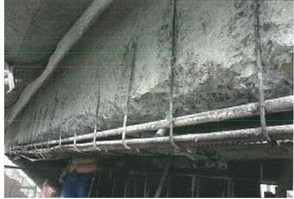
Figure (VIII-140) Damaged concrete cover removal from longitudinal slab beam
