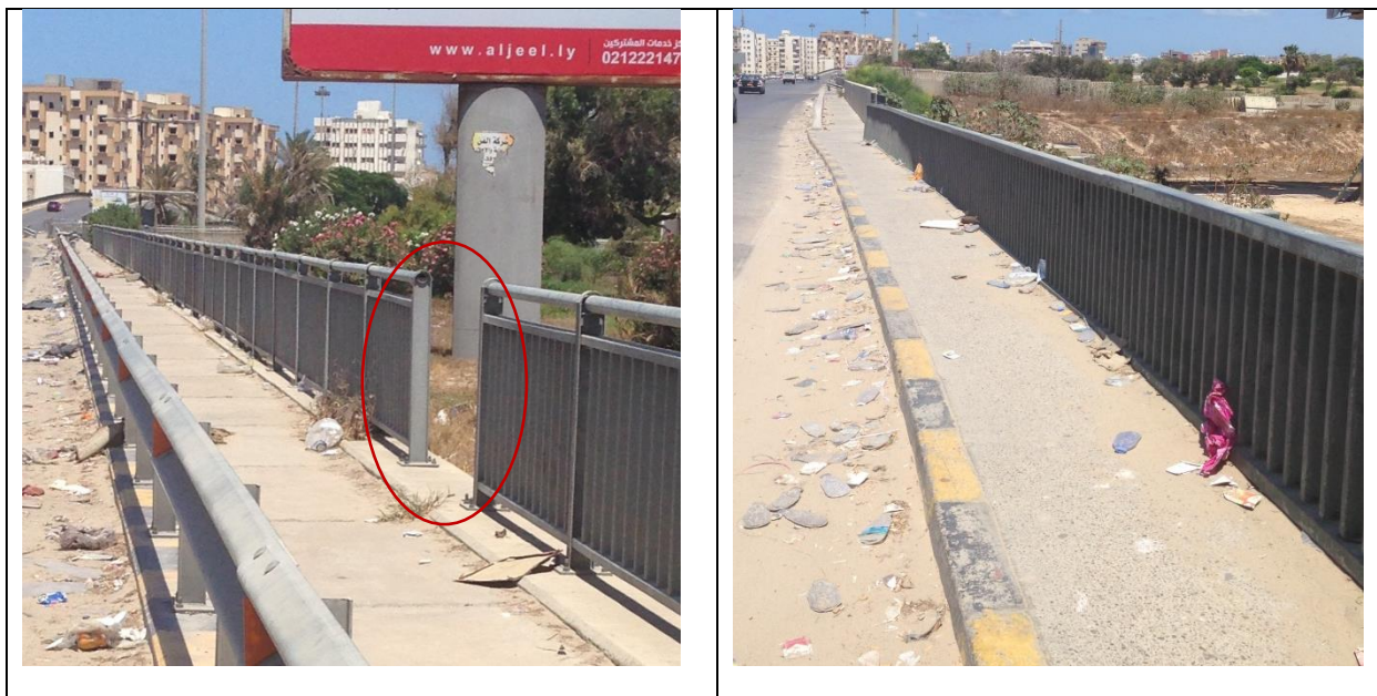
Figure (IX-17) A general view of fences on the bridge, with missing part
