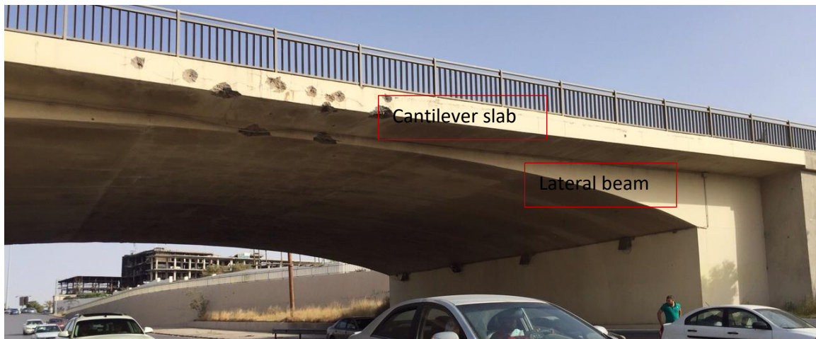
Figure (IX-26): A View of lateral beam of arch slab, and cantilever slab, middle part
