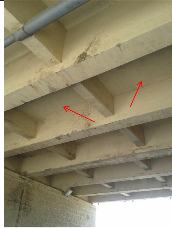
Figure (IX-92) View of deck slab with support walls, longitudinal and transversal supporting beams
