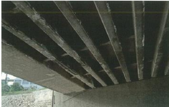
Figure VI-145. Damaged main beams: dark and white steins, reinforcement corrosion, spalling of concrete cover
