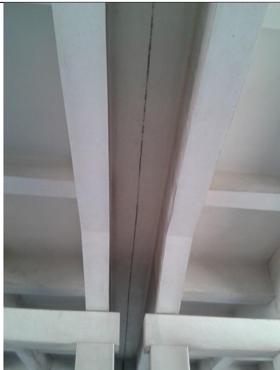
Figure (IX-146) A general view of expansion joint between deck slabs in superstructure of bridge
