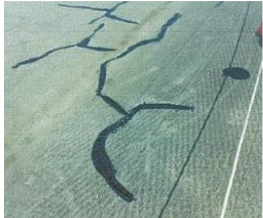
Figure (VIII-43) View of cracks after injection
