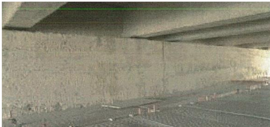
Figure Vi-164. Damaged upper part of abutment: deep spalling off of cover
