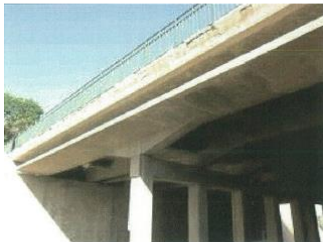
Figure Vi-165. Beam for fence with damaged concrete
