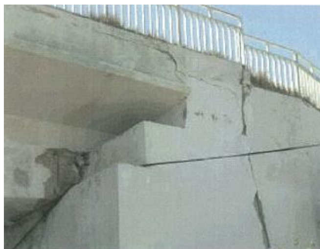
Figure VI-105. Damaged plaster and concrete next to the interior wall
