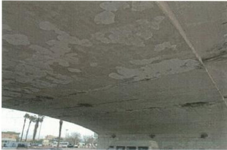
Figure VI-53. Deck ceiling, falling off painting and plaster layer, damage of concrete due to corrosion of reinforced bars
