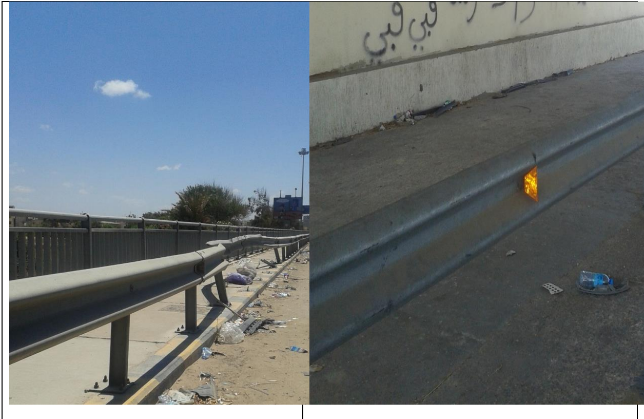
Figure (IX-41): General view of the guardrail on the bridge with damage
