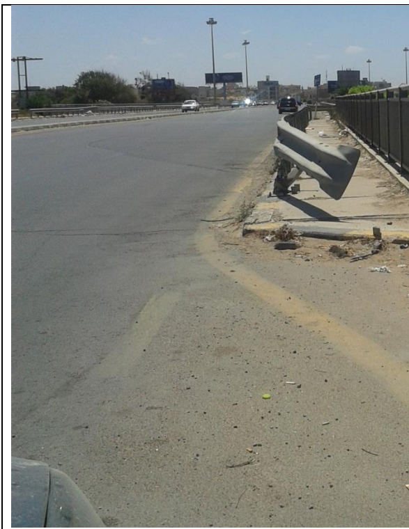
Figure (IX-37): A general view of asphalt wearing layer, transversal crack
