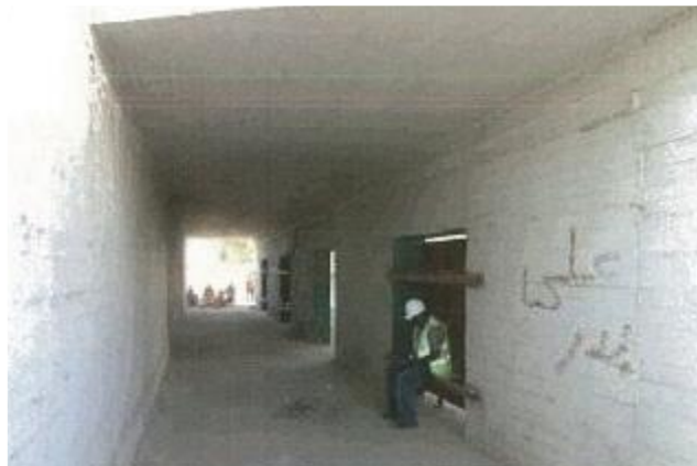
Figure VI-85. Tunnel between the interior wall and exterior wall, uneven concrete surface
