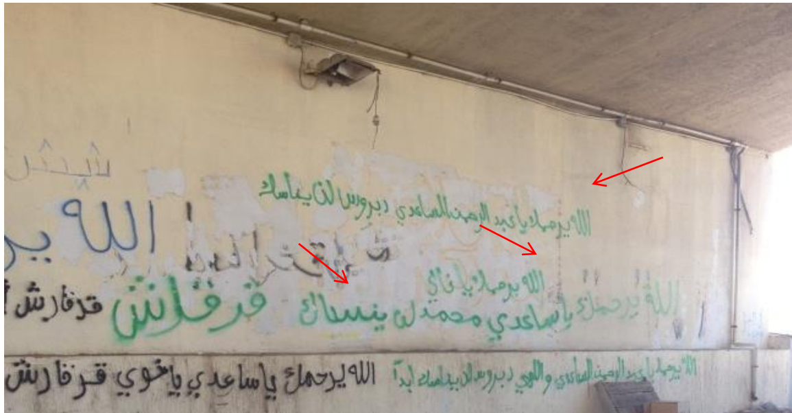
Figure (IX-14) Cracks in supporting wall
