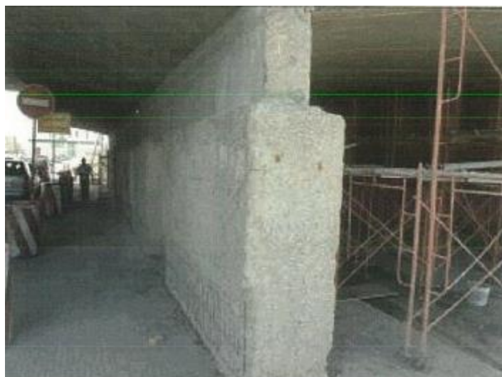
Figure (VIII-102) Supporting wall with damaged concrete removed and exposed reinforcing bars
