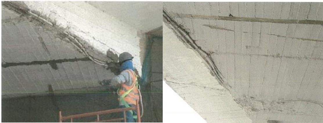
Figure VI-82. Bared, deformed and twisted reinforced bars in ceiling beam
