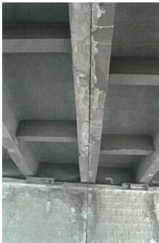
Figure VI-130. Joint between two deck slabs: water leakage, spalling of mortar layer, white and dark stains
