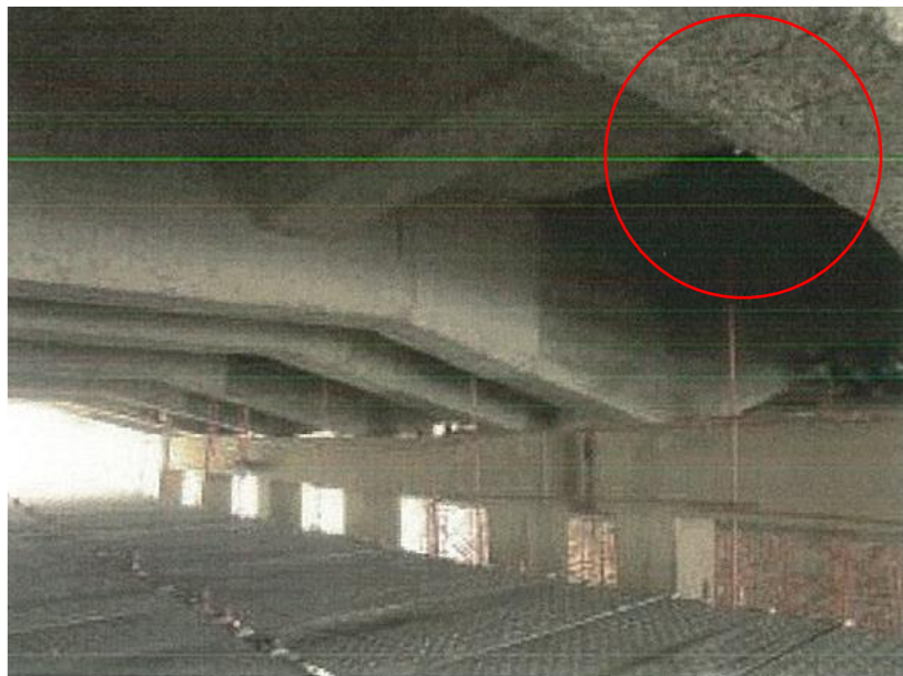
Figure VI-168. Damaged deck ceiling beams, exposed rebar, thin cover, spalling off of cover
