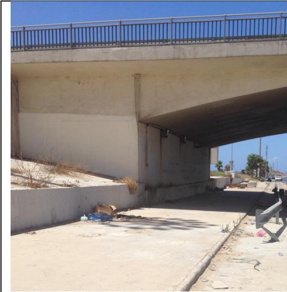
Figure (IX-3) A View of supporting part of lateral beam of arch slab, east side.
