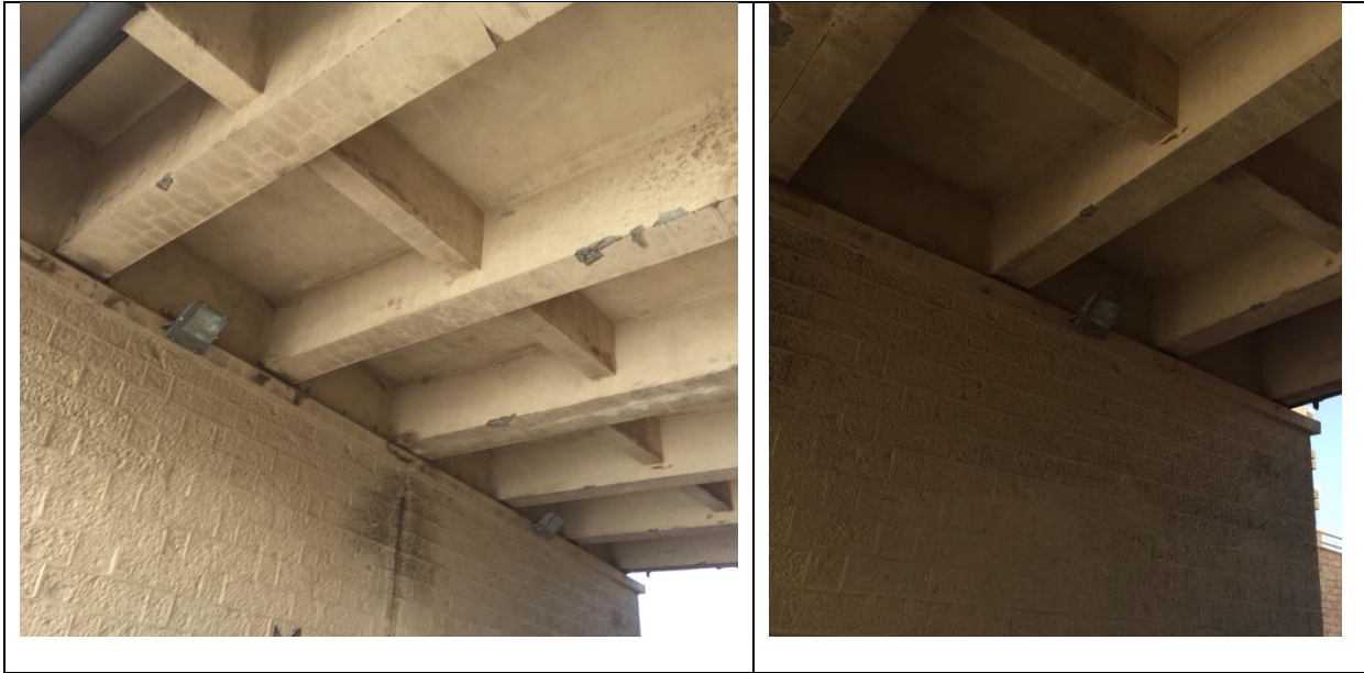
Figure (IX-94) Longitudinal and transversal supporting beams, net like cracks, corner spalling off, traces of dust
