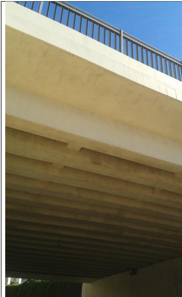
Figure (IX-115) A view of cantilever slab lateral and lower part (north side)
