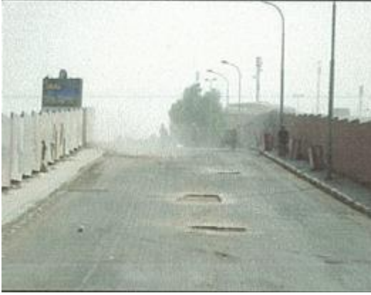
Figure (VIII-90). A view of old asphalt layer on the bridge before removing of surface layer
