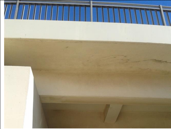
Figure (IX-145) A general view of down part of cantilever of superstructure of bridge
