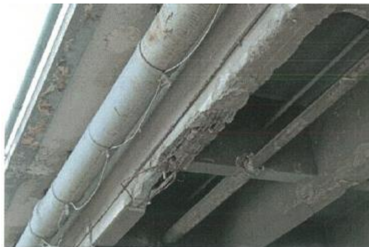
Figure VI-129. Damaged external longitudinal beam: bared, deformed and twisted rebars, crashed and cracked concrete reinforced in beam: spalling of mortar from cantilever slab
