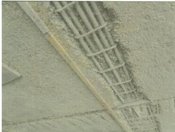
Figure (VIII-14) Rebars protective coating and leveling ribs of wood ready for application of cementitious base special mortar
