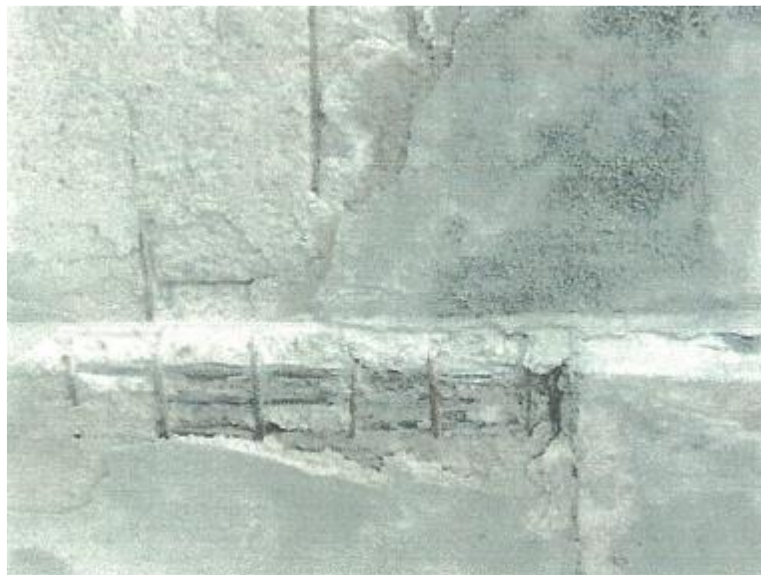
Figure VI-23. Exposed reinforced bars in lateral beam of arch slab, and in cantilever slab. Corrosion of bars, falling down of cover and plaster layer
