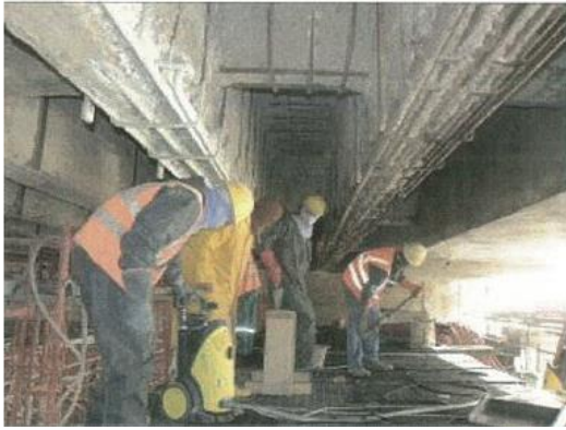
Figure (VIII-162) Removal of damaged concrete and rebars cleaning with water-sand blasting, longitudinal slab beam
