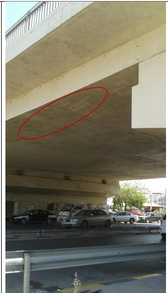
Figure (IX-70) View of deck slab, down side of cantilever slab with support walls, net like crack
