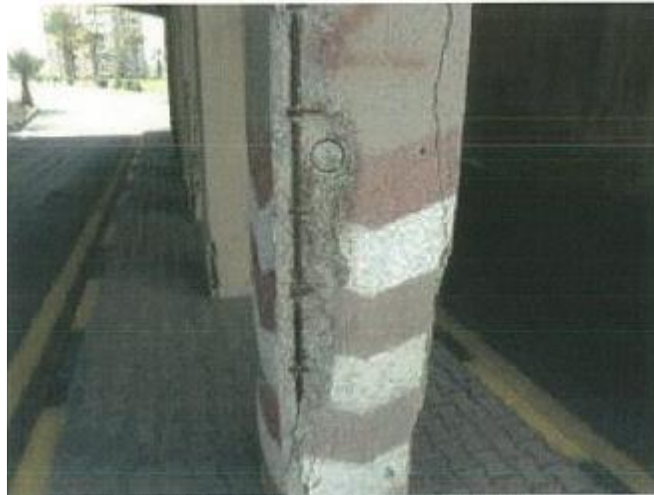
Figure Vi-163. Cracking of cover in support column, spalling off corner concrete
