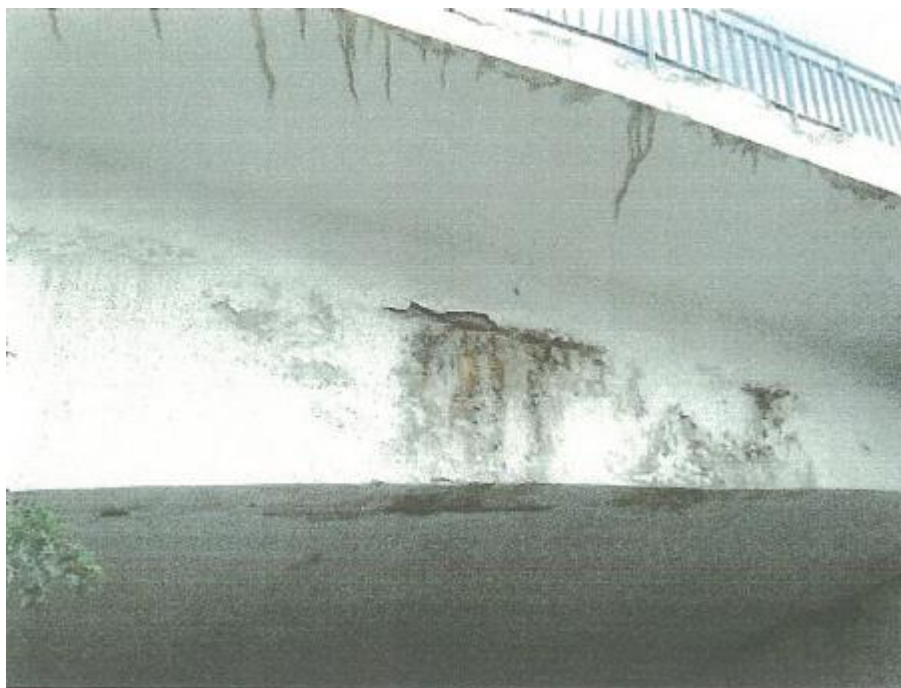
Figure VI-110. Traces of leakage water on lateral beam and cantilever slab, corrosion of rebars, spalling of plaster, pilling off of paint
