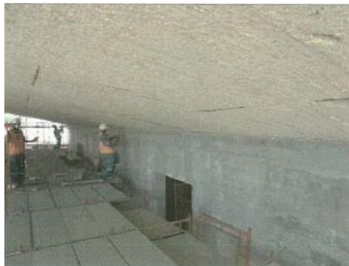
Figure (VIII-73) Damaged concrete cover removal from ceiling beams
