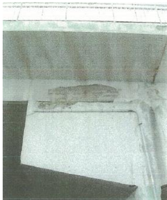
Figure VI-109. Spalling of plaster on deep supporting element
