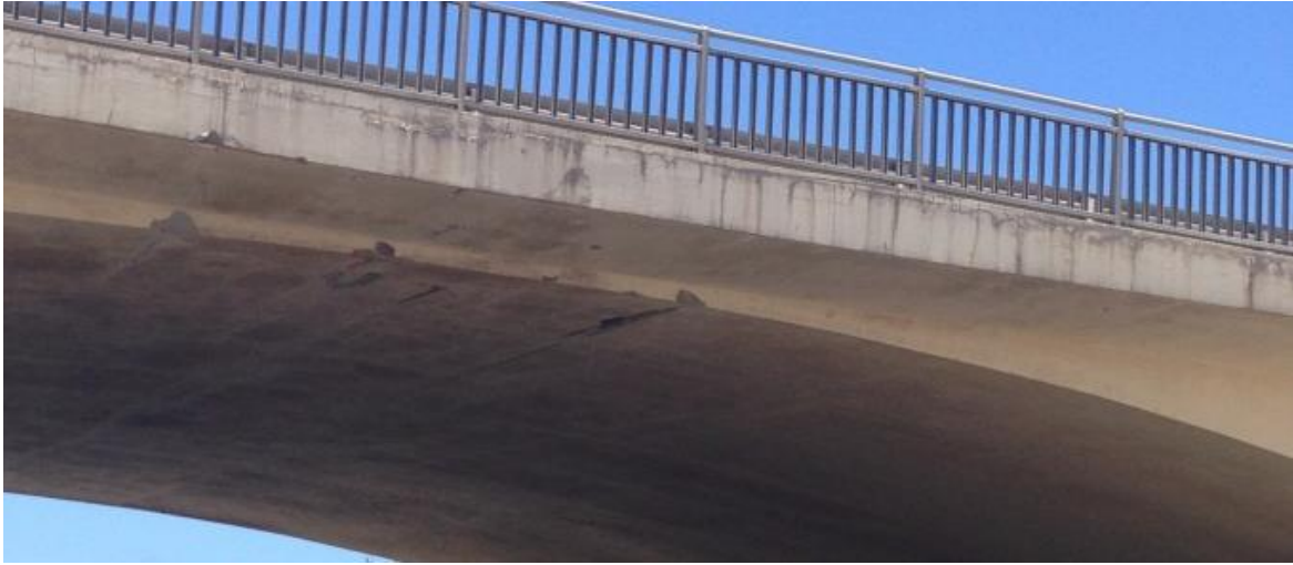
Figure (IX-11) The characteristic damages on side surface of cantilever slab
