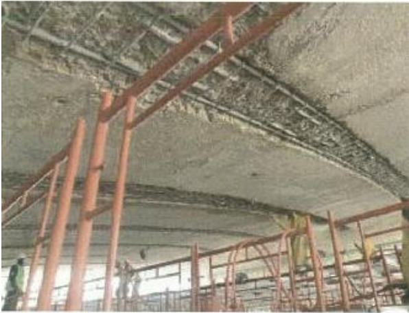
Figure (VIII-63) Covering the rebars on ceiling beams with cementitious base protection
