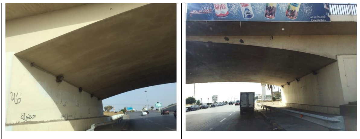
Figure (IX- 24): A view of supporting part of lateral beam of arch slab, east side
