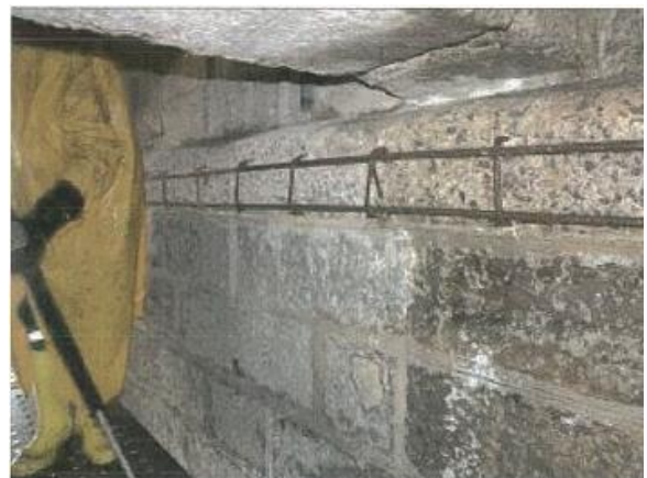
Figure (VIII-143) Cleaning of rebars with water-sand blasting, top beam of the support wall
