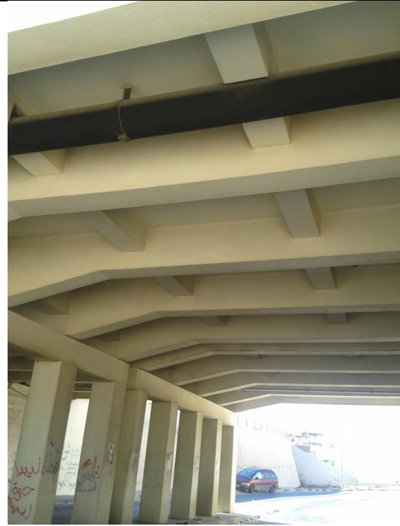
Figure (IX-141) A general view of main and secondary beams of superstructure of bridge
