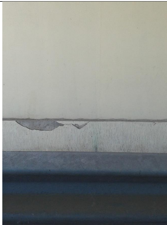
Figure (IX-32): Supporting Wall, the detail of damage of plinth
