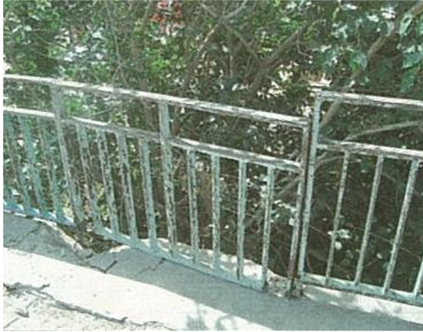
Figure VI-86. Damaged and corroded old fence and damaged part of side walk
