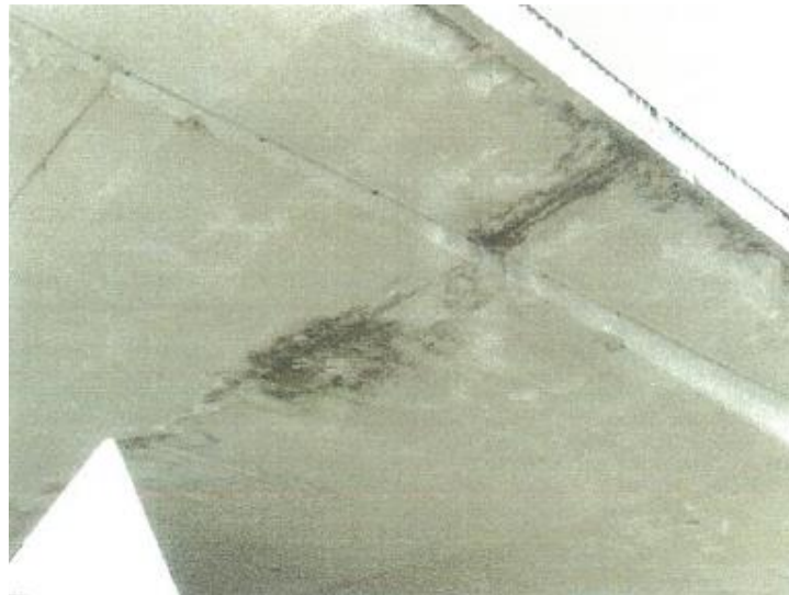
Figure VI-24. Leakage of water through cantilever slab and through joint between arch slab and simple supported beam slab, damaged edge of cantilever slab (edge beam)
