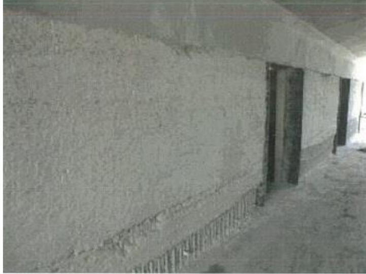
Figure (VIII-103) General view of the supporting wall with damaged concrete removed and exposed rebar
