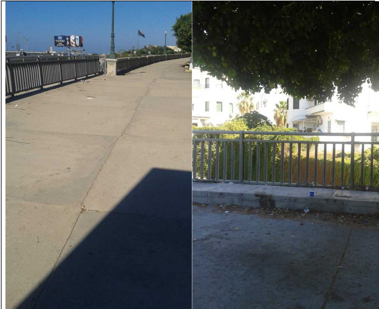
Figure (IX-121) A general view of pedestrian path on bridge (north side)
