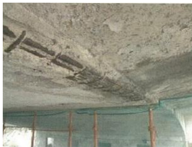
Figure VI-26. Exposed reinforced in beam slab next to the cantilever, corrosion of bars, falling down of cover and plaster coating
