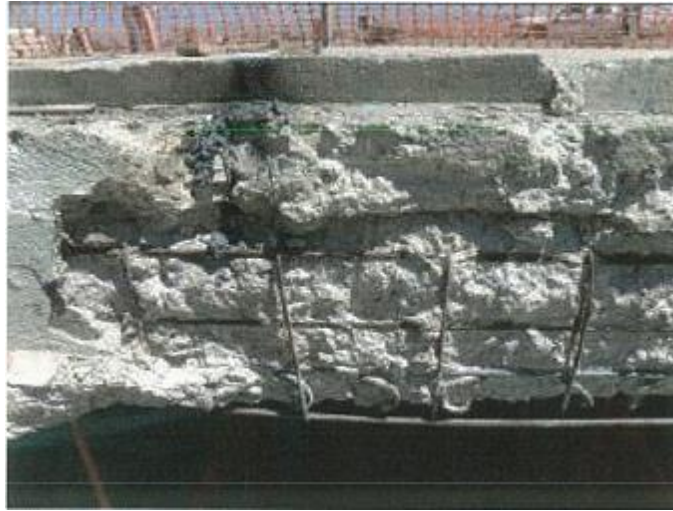
Figure VI-111. Bad adhesion between reinforced bars and concrete (cantilever slab)
