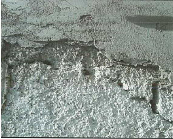
Figure (VIII-113) A very large crack in abutment wall
