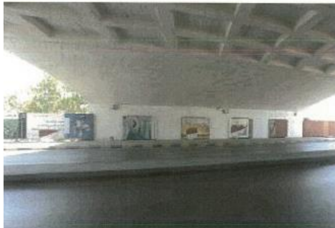
Figure VI-79. Desk ceiling, pilling off painting cover
