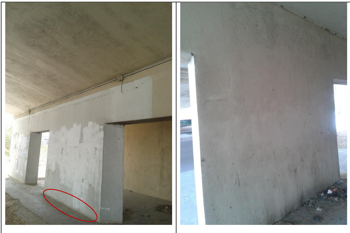
Figure (IX-51) View of supporting wall with ceiling, peeling off protective painting
