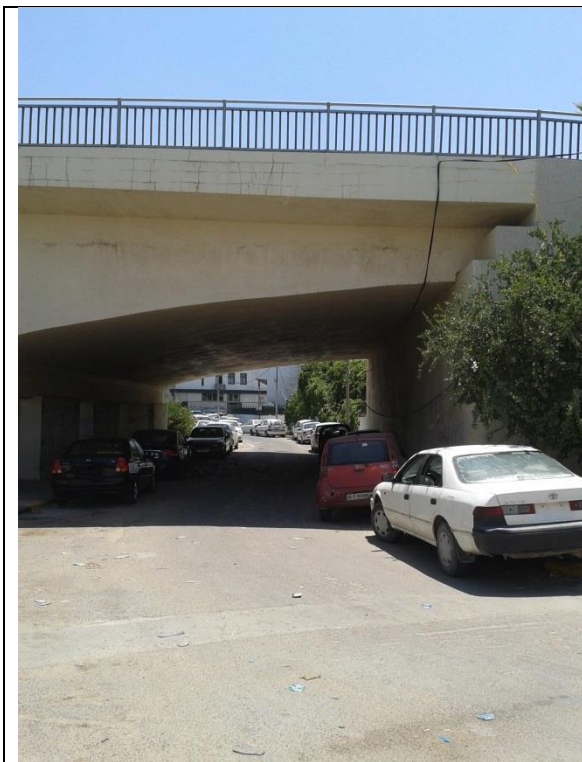
Figure (IX-67) A general view of Bab Bin Gheshir road bridge, side part, west
