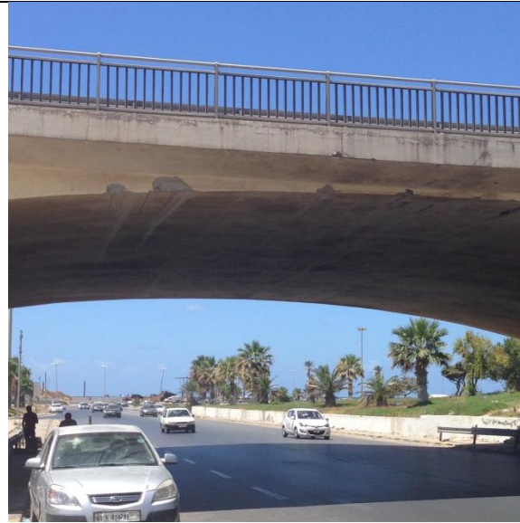
Figure (IX-4) A View of lateral beam of arch slab and cantilever slab, east side.
