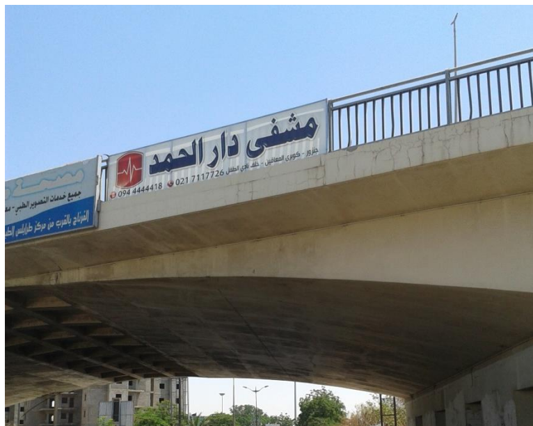
Figure (IX-50) View of cantilever slab, vertical and horizontal cracks
