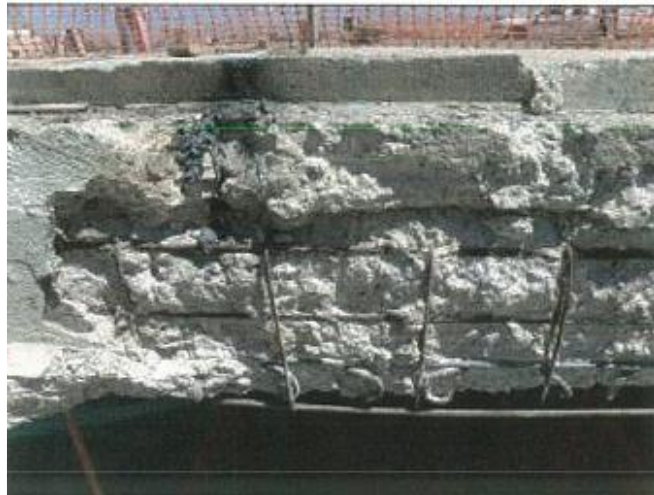
Figure (VIII-106) Corroded steel on the cantilevers
