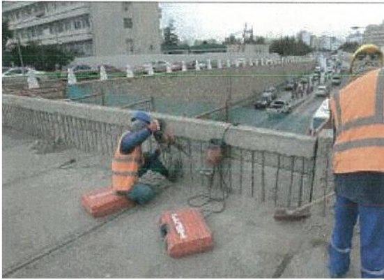
Figure (VIII-139) Damaged cover removal from concrete part of fence, top of the bridge
