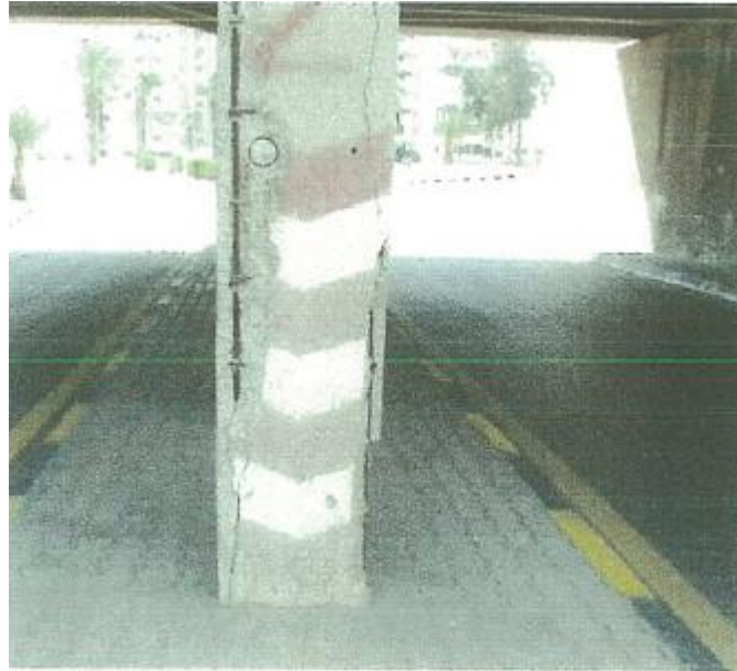
Figure VI-161. Damaged column: Exposed reinforcement bars, corrosion of rebar, cracking of concrete along the edge rebar, spalling off corner concrete
