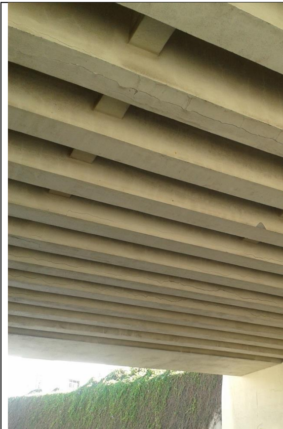
Figure (IX-113) Longitudinal and transversal supporting beams, longitudinal and transverse cracks in longitudinal beams, spalling off, traces of dust
