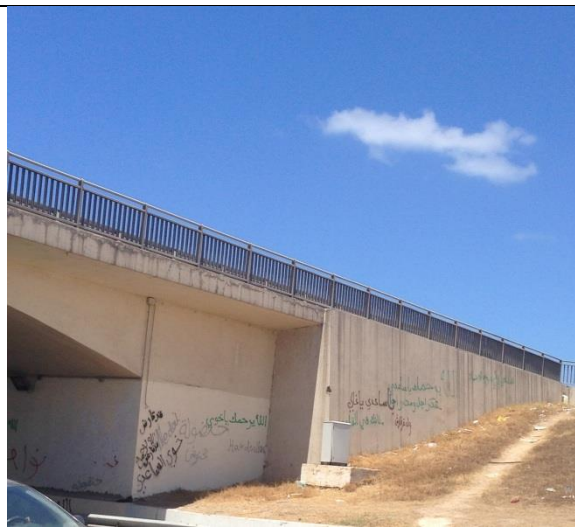
Figure (IX-6) A View of supporting part of lateral beam of arch slab, west side
