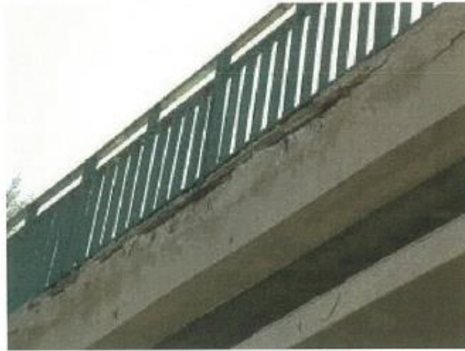
Figure VI-166. Beam for fence: Corrosion of reinforcing bars, insufficient depth of cover, cracking and falling off of concrete cover, water stains due to overflow of water over the edge of the beam
