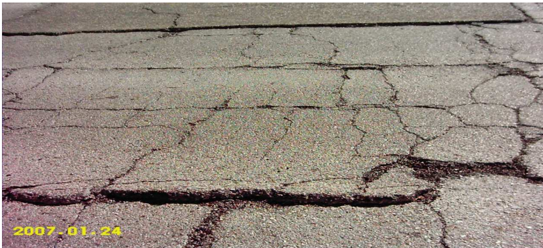
Figure 3.6 Alligator cracking distress in Libyan roads
