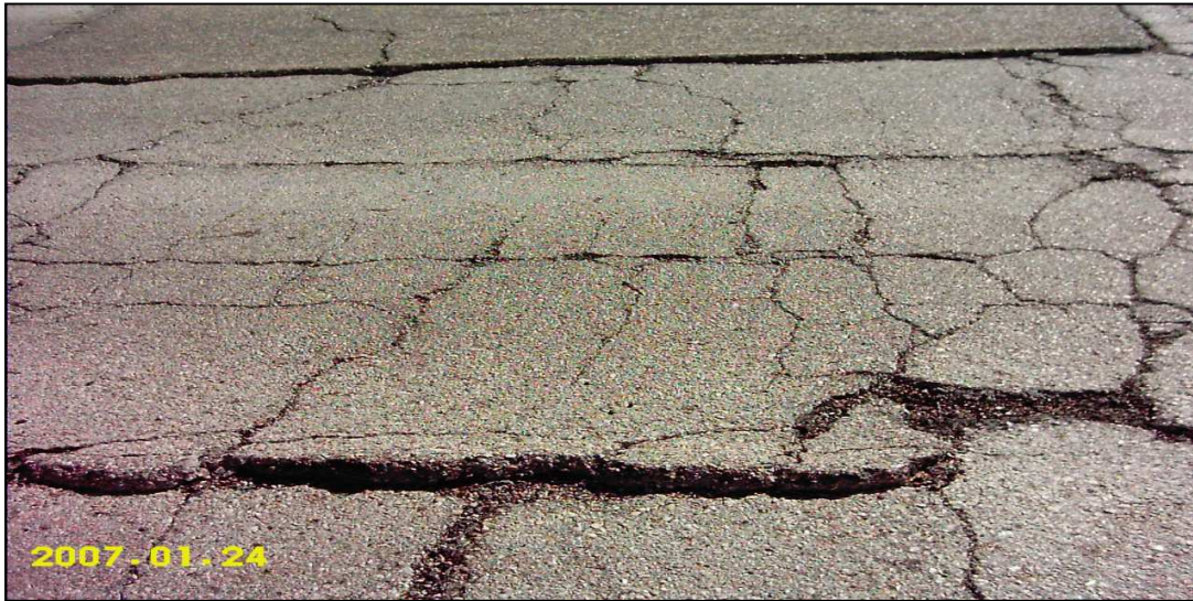
Figure 3.7 Alligator cracks in Libya roads
