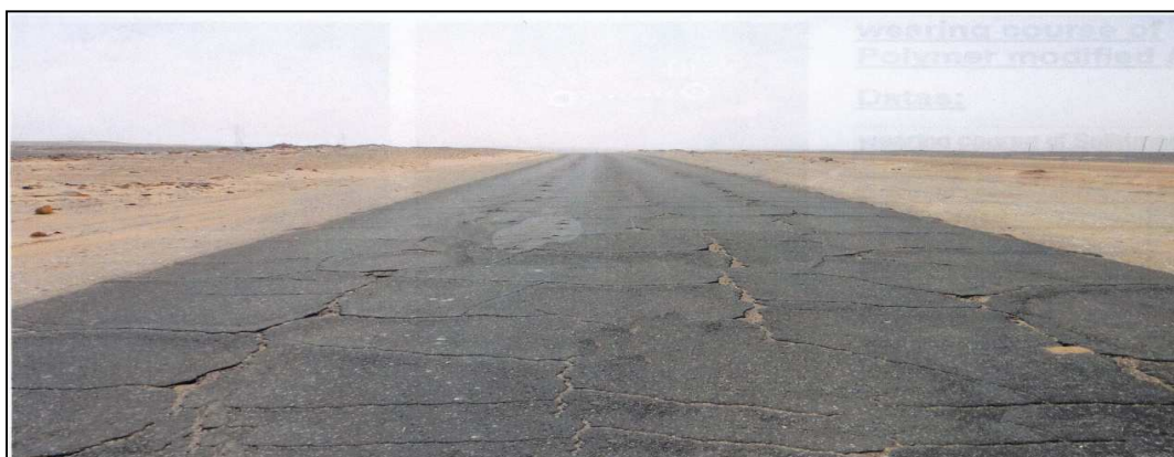
Figure 3.4 Block cracking distress in Libyan roads
