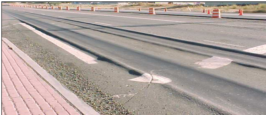
Figure 3.10 Rutting distresses ( http://www.pavementinteractive.org/article/rutting/ )
