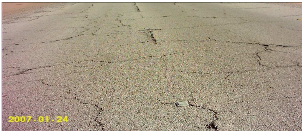
Figure 3.11 Road damages in Libya roads
