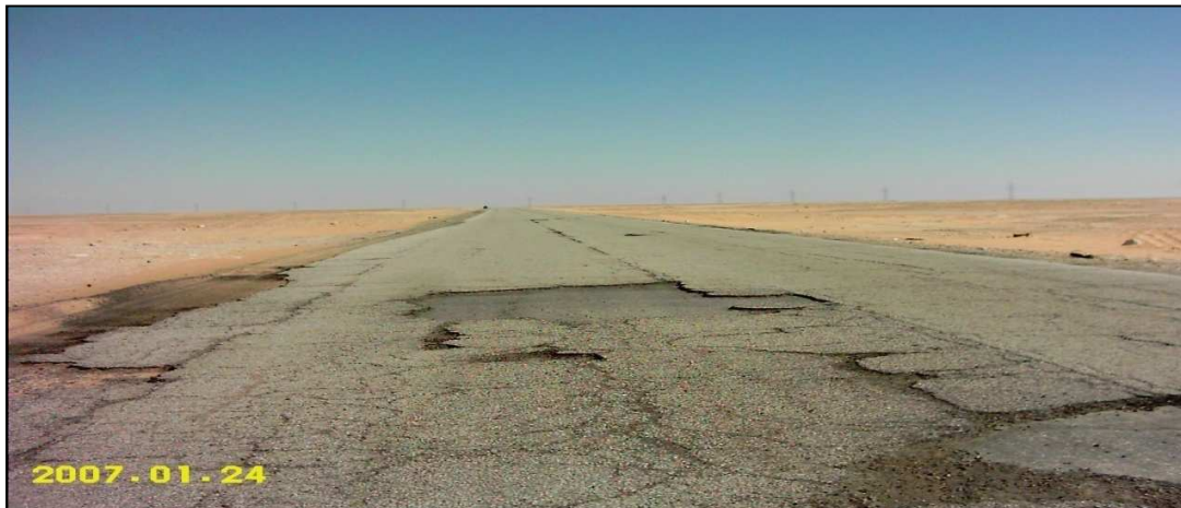
Figure 3.9 Road damages in Libya roads
