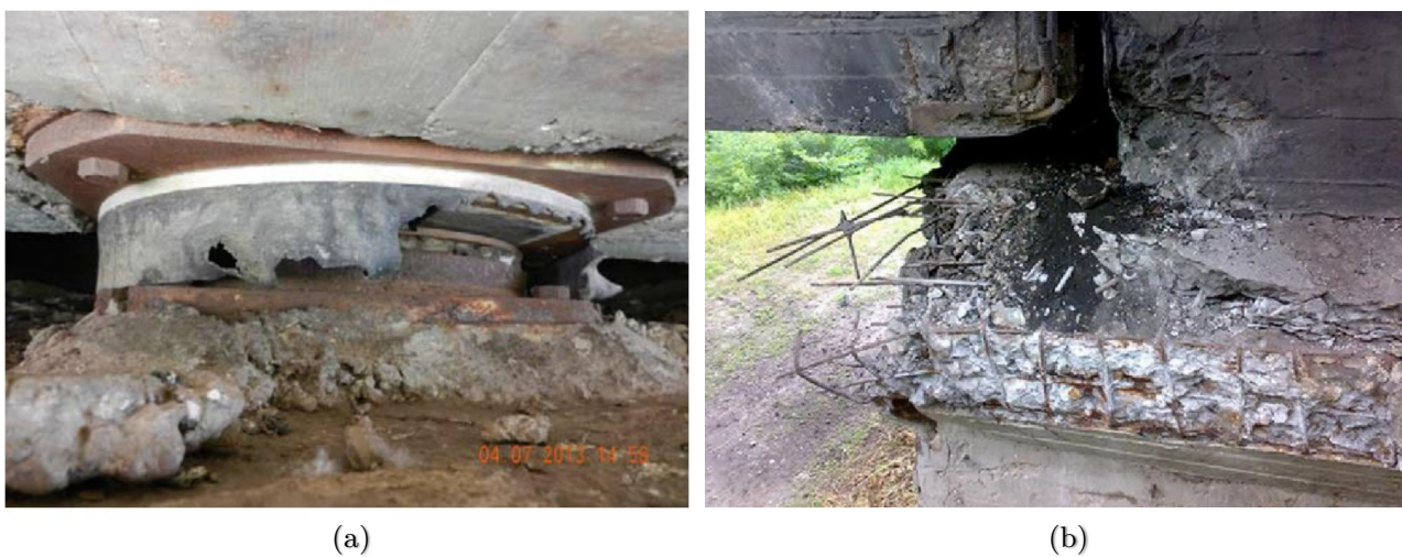
Figure 2.5. Damage of bearing area: (a) Corroded steel and demolished rubber of the bearing, (b) Large spalling on the abutment and the girder end.
