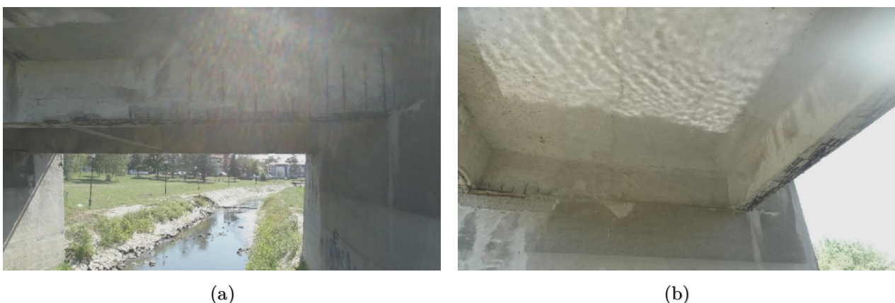
Figure 5.5. (a) Oversaturated photo of the bridge, (b) water reflection on the bridge deck.
