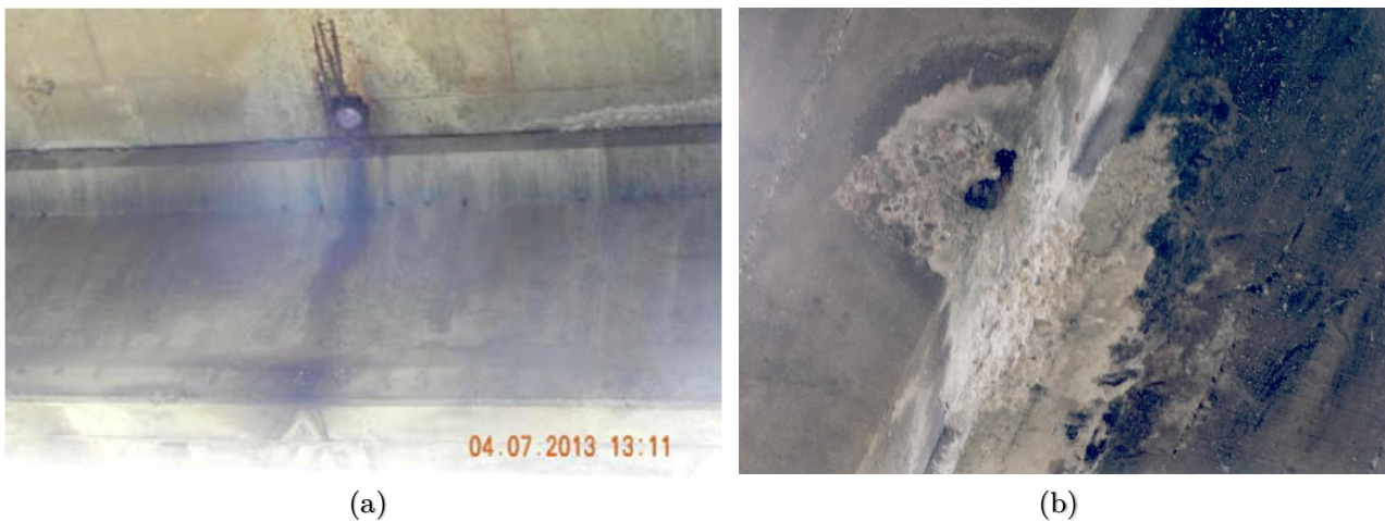
Figure 2.4. Damage induced by degraded drainage pipe: concrete deterioration in its (a) initial and (b) advanced phase.
