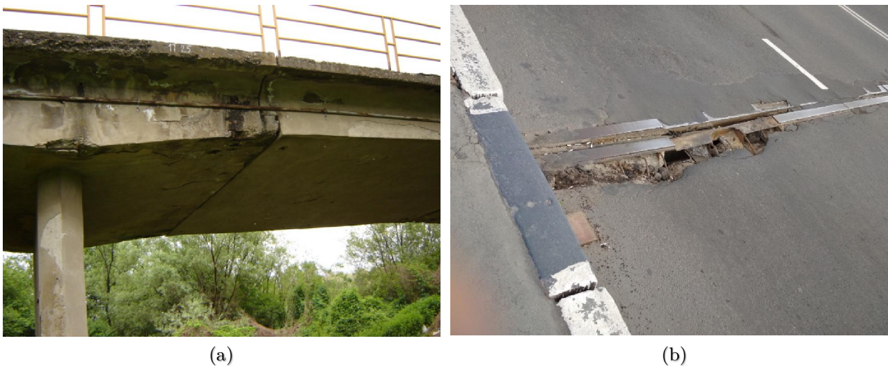
Figure 2.2. Damage due to the water penetration between elements: (a) Spalled ends of deck elements in the joint, (b) Detached pavement from the dilatation mechanism.
