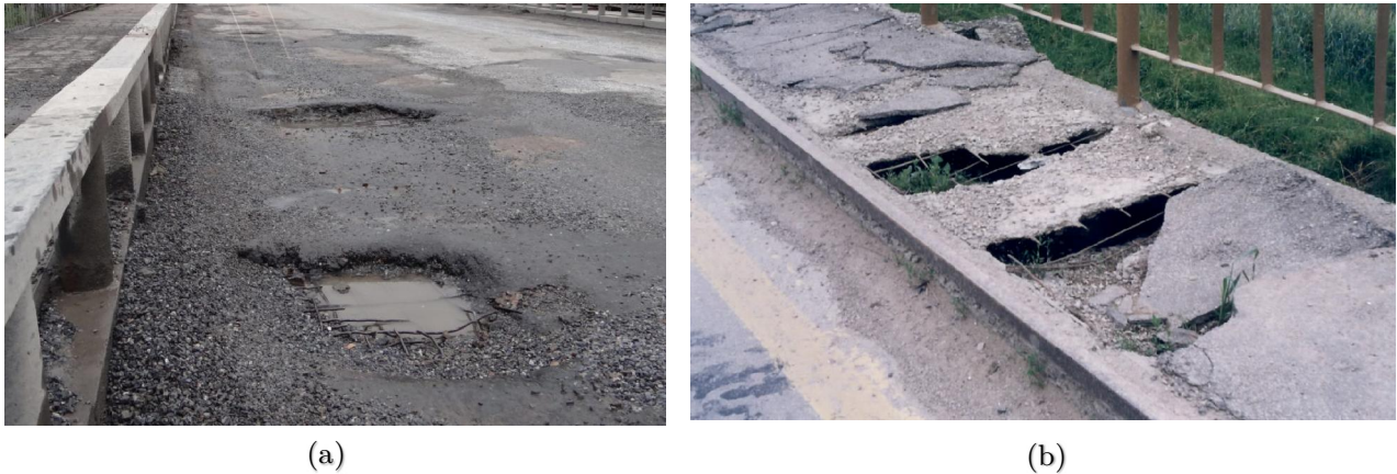
Figure 2.3. Damage of mainly horizontal elements under high dynamic load: (a) Pavement hole, (b) Completely deteriorated sidewalk structure.
